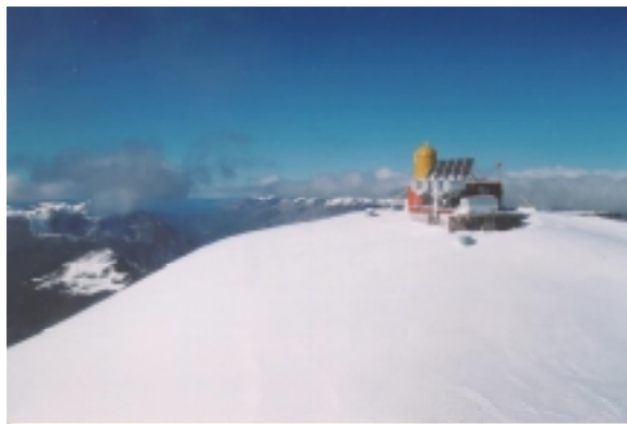
Figure 1. This PV-hybrid telecommunication station owned by NorthwesTel is being studied as part of the Canadian PV-hybrid R&D program at CANMET-EDRL.
